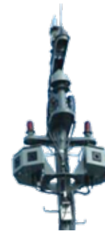
Installed split ESM antenna array
