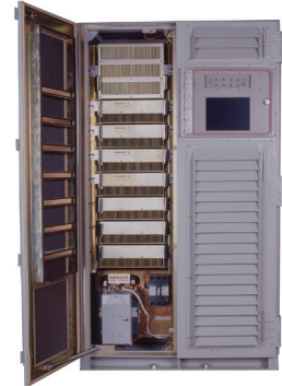
Partial interior view showing rectifier and inverter modules
